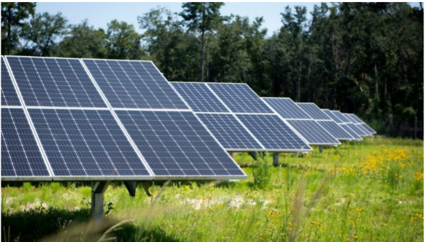
This array of solar panels at Moody Air Force Base, Georgia, saves $700,000 annually. (Department of the Air Force photo by Airman 1st Class Megan Estrada)
